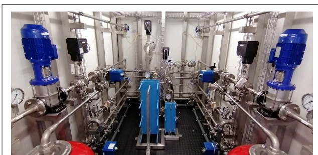
Fig. 2: Example of a containerized heat transfer station to meet the requirements of the chemical industry
